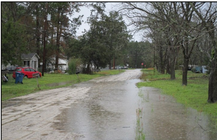
The Emerson Park area of Ware County's Street Paving and Drainage improvements will include six safe, paved roads on which to travel, and a functioning storm drainage system to efficiently remove rainwater from the neighborhood.
