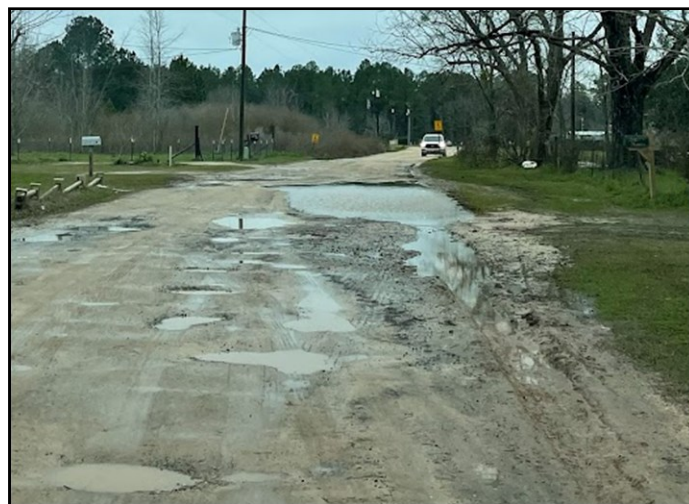
Harrell Road will be improved with CDBG funds in Cook County. Upon completion of the project, residents will no longer be endangered by this frequently flooded roadway.
