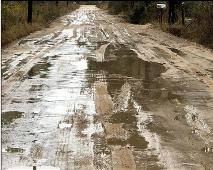
Pictured here is the street that will be improved with CDBG funds in Berrien County. Upon completion of the project, residents will no longer be endangered by this frequently flooded roadway.
